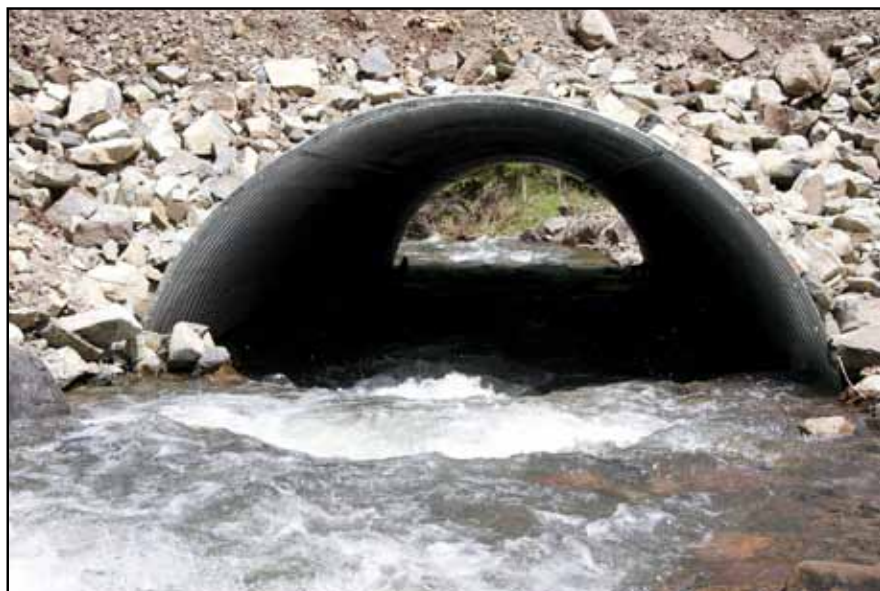
Adequately sized culverts are essential to preventing road wash-out and allowing for fish passage.
